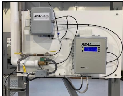
UVT Analyzer – tells the UV Reactor what intensity the lamps need to be.
